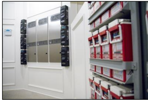
Fig. 1: A hybrid inverter system in a residential installation. Hybrid inverters work with batteries to store power
