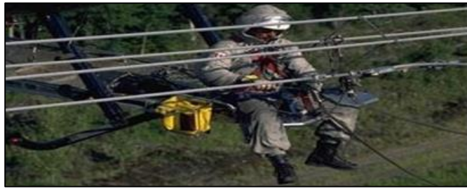
Fig. 3: Replacement of failed splice
