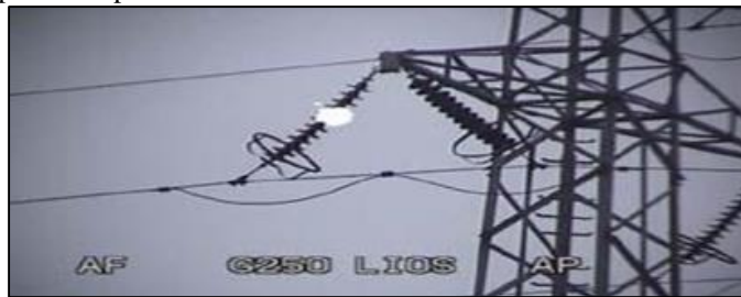
Fig. 4: Corona on failing porcelain insulator
