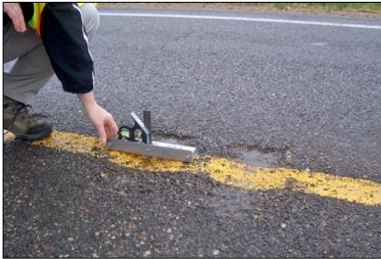
Fig. 2: Deterioration of pavement surface due to stripping distress. http://www.pavementinteractive.org/article/raveling/
