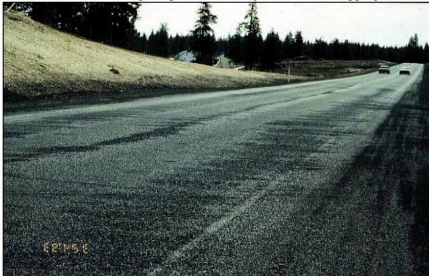
Fig. 1: Effect of stripping distress on HMA pavement layer. http://safety.fhwa.dot.gov/roadway_dept/pavement/rumble_strips/faqs.cfm
