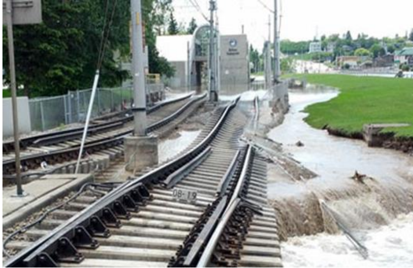
Fig. 2: Damaged LRT tracks over the Elbow River between Erlton and stampede station. Calgary, 2003 Source: https://www.tumblr.com/search/Calgary-flood
