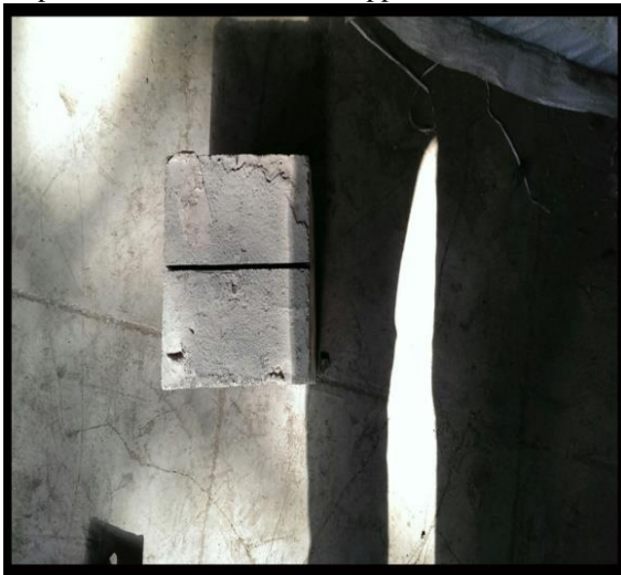
Fig. 1: Crack made of 15 mm depth
